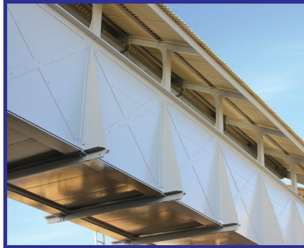
Dawlish Station footbridge uses a combination of pultrusions and resin infusion to replace a listed iron bridge designed by Brunel. Courtesy of Tony Gee and Partners
